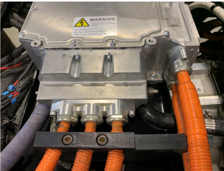
Inverter with high voltage label, secured orange HV cables and cooling unit
