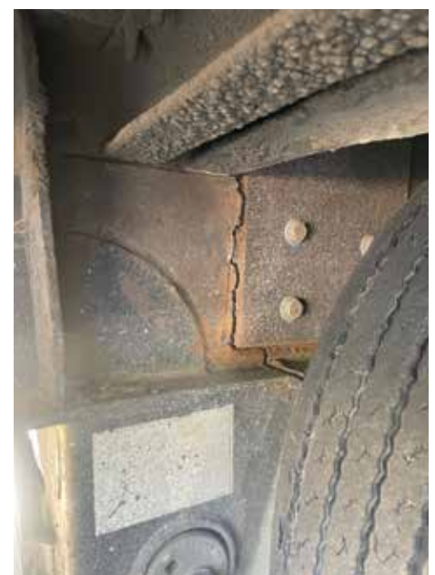
At the multi-agency inspection detail in Midlothian, Texas, inspectors discovered this cracked frame, which was on a trailer loaded with flattened cars with a total of 75,000 pounds gross weight.
