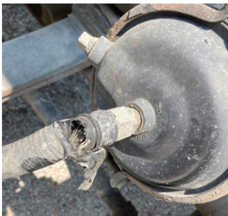
Hole in brake chamber hose.
