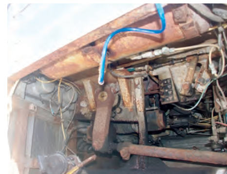
PICTURE #3: The final connection from compressor to air supply tank, which is a pretty sly fix, yet completely unsafe and against regulation.
