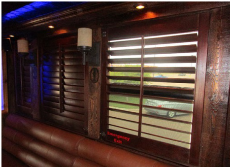
Exit obstructed by wooden plantation shutters.
