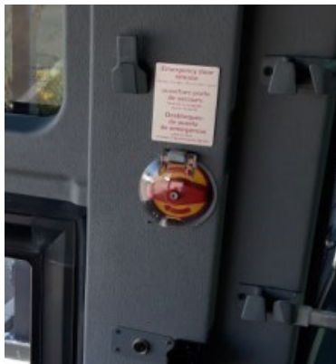
Door release valve inside a motorcoach at the entrance door.
